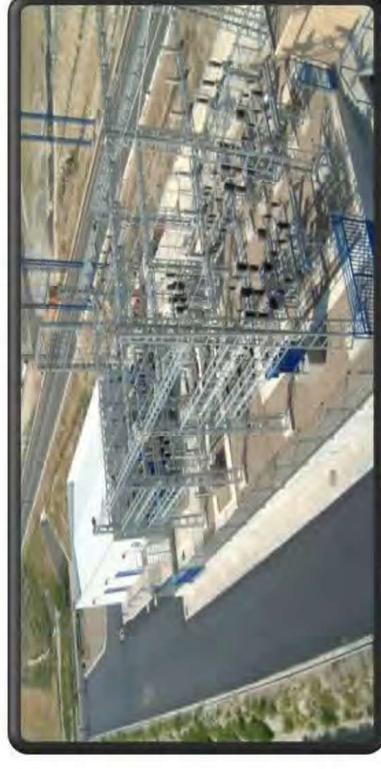
Example: Traction Power Facility
