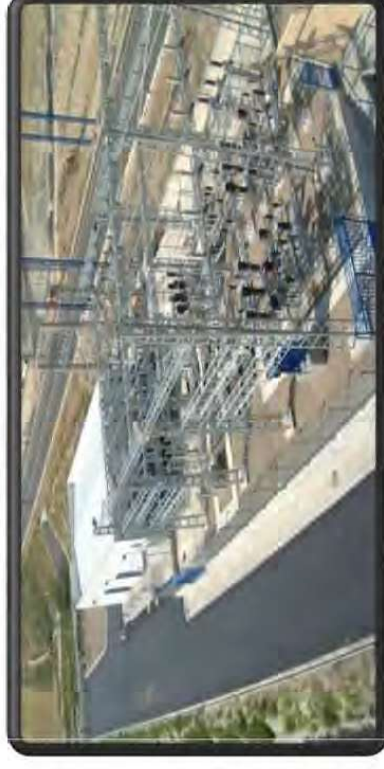
Example: Traction Power Facility
