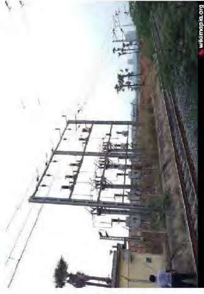
Traction Power Switching Station
