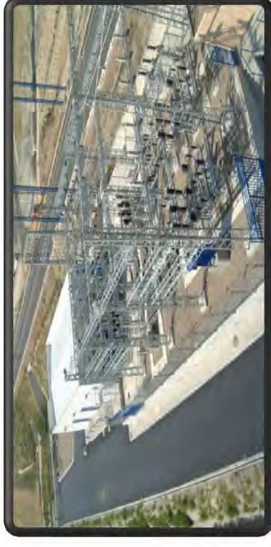
Example: Traction Power Facility
