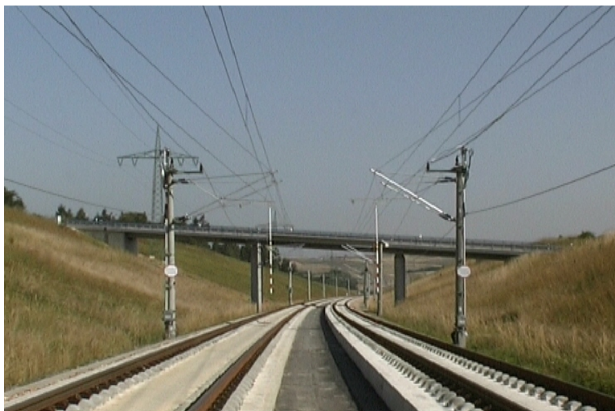
FIGURE 2-2: CATENARY ON THE COLOGNE – FRANKFORT HIGH SPEED LINE
